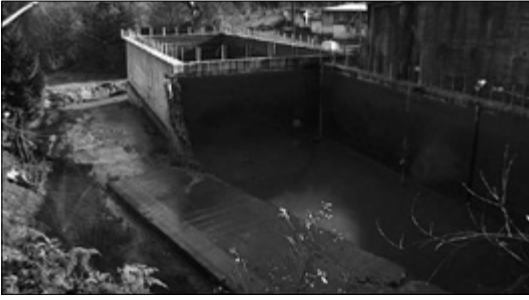
Il. 2. Collapsed effluent tank
