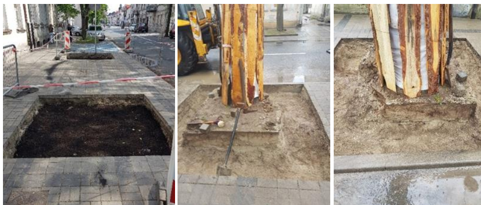
Fig. 4. Photos from the replacement of the pavement around trees on Kazimierza Wielkiego Street in Płock
